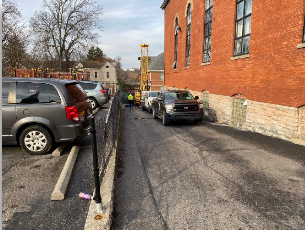
Photograph 4: Drilling Boring B-3. Concrete retaining wall providing grade separation from parking lot.
