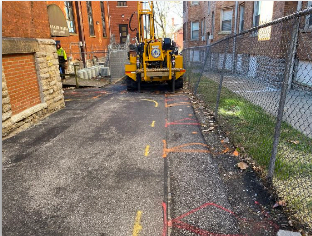
Photograph 6: Drilling Boring B-2. Existing underground utilities at northeast portion of the site.
